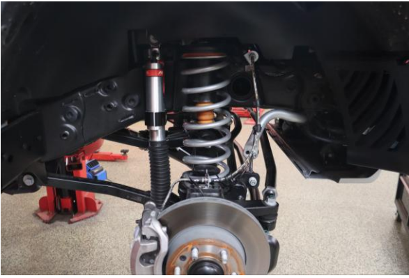
13. Release the spring compressors allowing the spring to sit in the upper isolator and lower perch.
