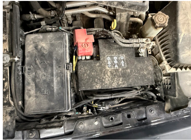
Fig. 39a: Connect 12V 5A and 12V 15 A to positive terminal; connect GND BATT to ground terminal
