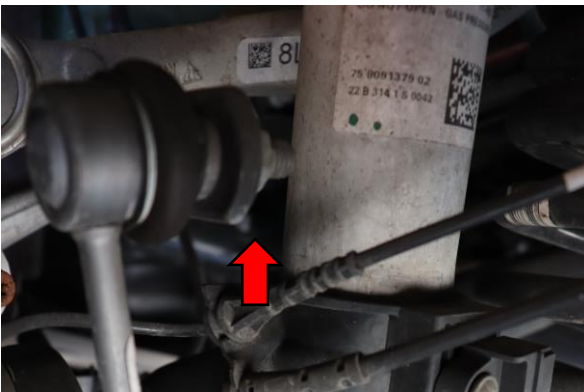
Step 17. Remove the left and right sway bar end link on the bar end using a 16mm and T30.
